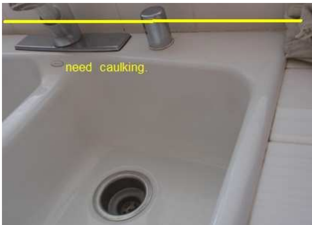
Around sink need caulking.
